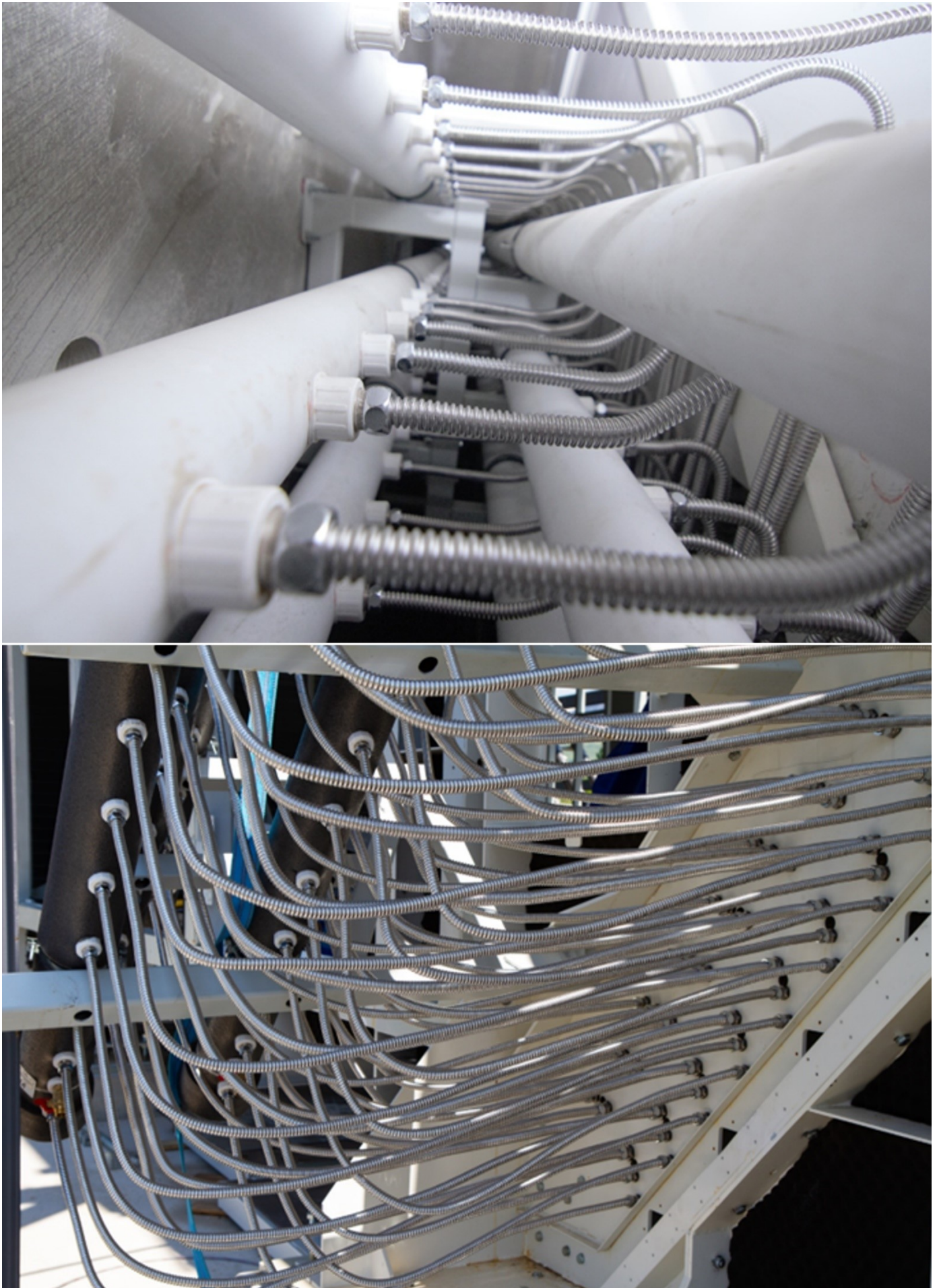
Fig. A.1.10 Custom manifolds.
