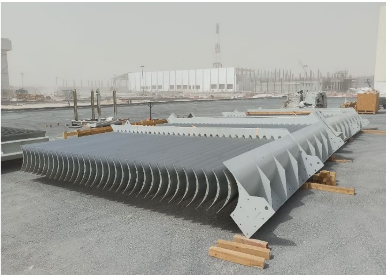
Fig. A.1.5 Turning vanes (TTE-TV) installed in the turning vane diagonal assembly (TTE-TSDA). A-side diagonal support has not yet been mounted during the wind tunnel construction process.
