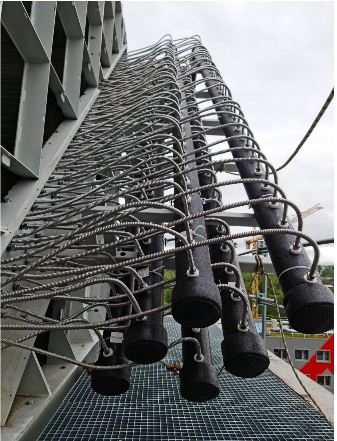
Fig. 2.10 Cooled turning vane manifolds and flexible hoses. Tunnel Tech PF45DL wind tunnel example. No casing. Top piping connection option.
